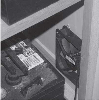
Ventilation fan draws in air
